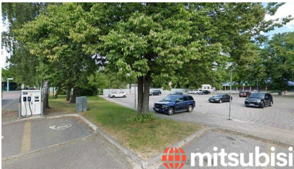
Csdd charging station ventspils
