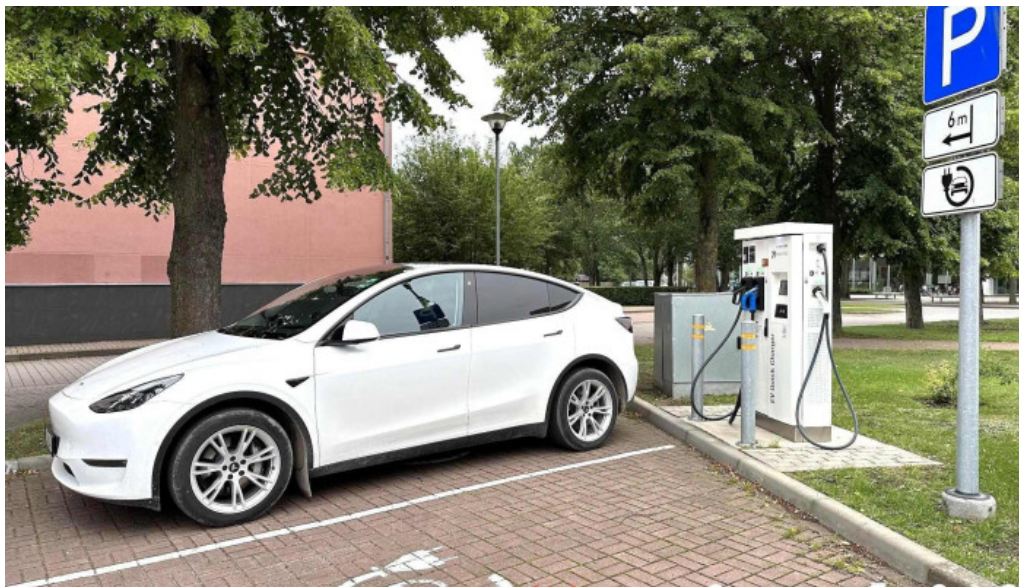
Csdd charging station visi
