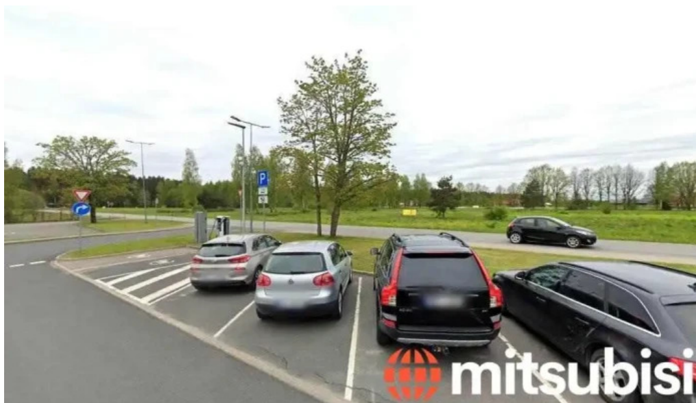
Be energised charging station valmiera
