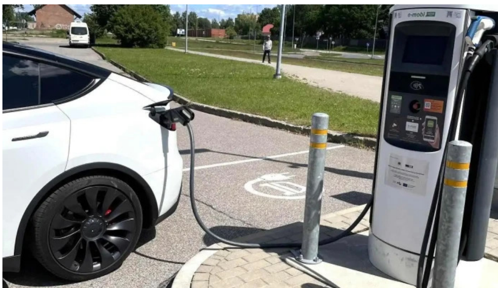
Fitek as charging station visi
