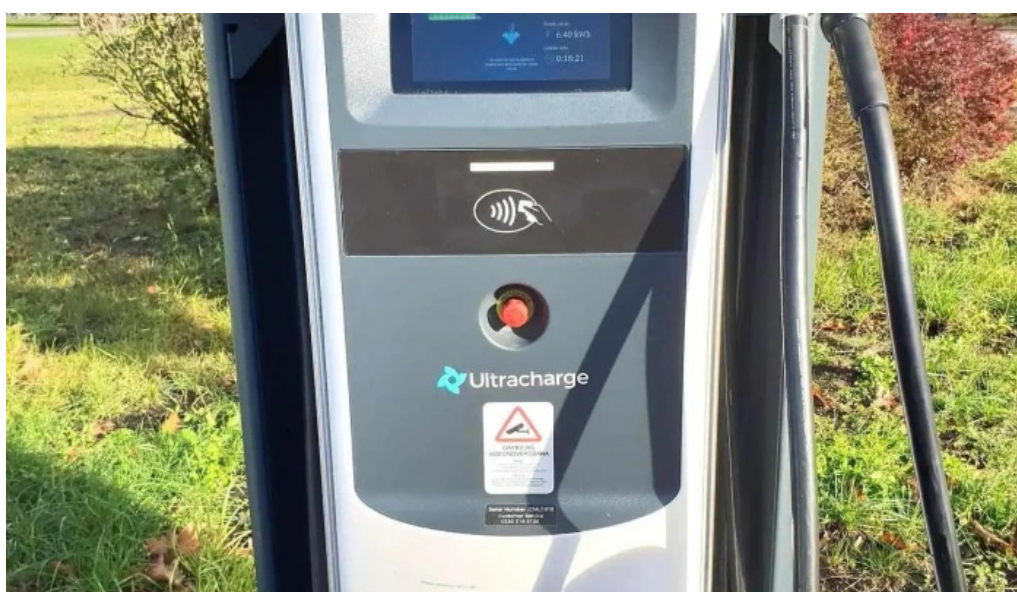
Csdd charging station visi
